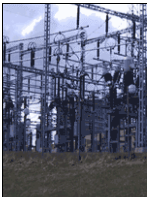
Fig. 10: Section 1 - The Power Plant
